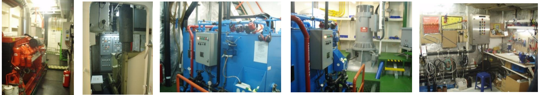
Additional aux engine room main deck, emergency gen, 50 men sewage treatment, bow thruster,
