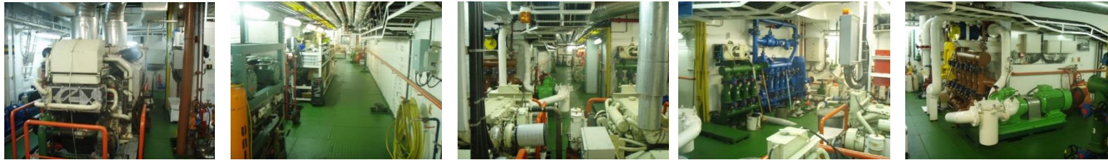
Engine room, 2 x Cummins QSK 60, various equipment, fuel / water manifold, 200 m3 fuel transfer pump
